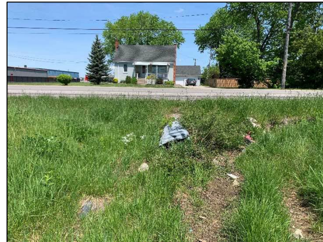
Photo 6. CSP culvert where the Intermittent Drainage Feature is conveyed beneath Killaly Street West onto the Subject Property facing north (24 May 2022).
